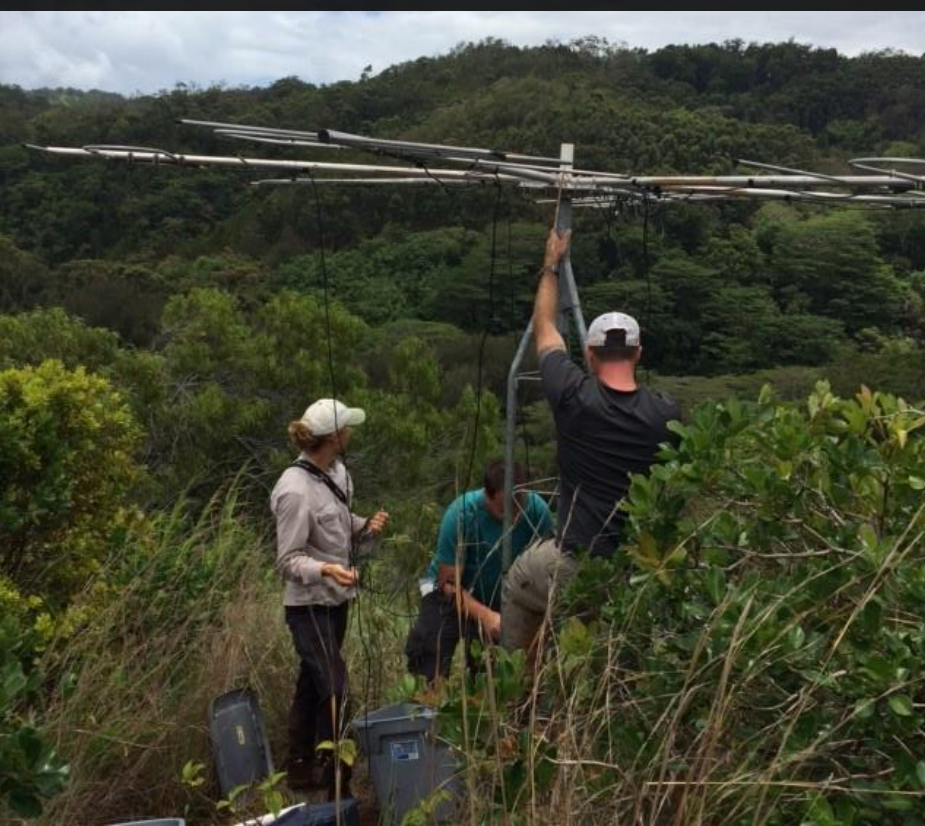
Scientists install a radio-telemetry tower in Oahu, Hawaii to track fruit-eating birds. The collected data showed how non-native species disperse native, endangered plants, 2015. (U.S. Army Corps of Engineers/Carmen Daugherty)
